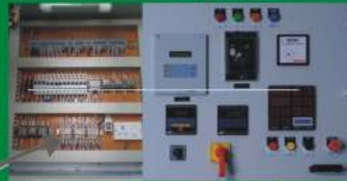
Metering & Internal Wiring
