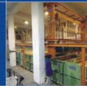
9 Tank Fully Automatic Pre-treatment
