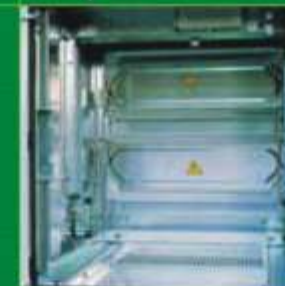
Shutter Assembly 33KV
