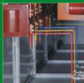
CT & Cable Compartment
