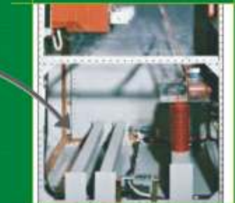
CT & Cable Compartment
